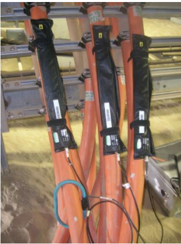
Example of FMC on medium voltage cables
